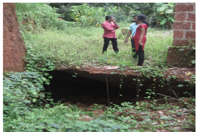
Fig. 1 Piping erosion observed in Kasaragod, Nelliyaadukkam
