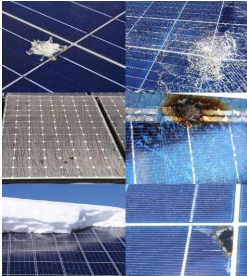
Fig. 2. Common Defects in Photovoltaic Panels
